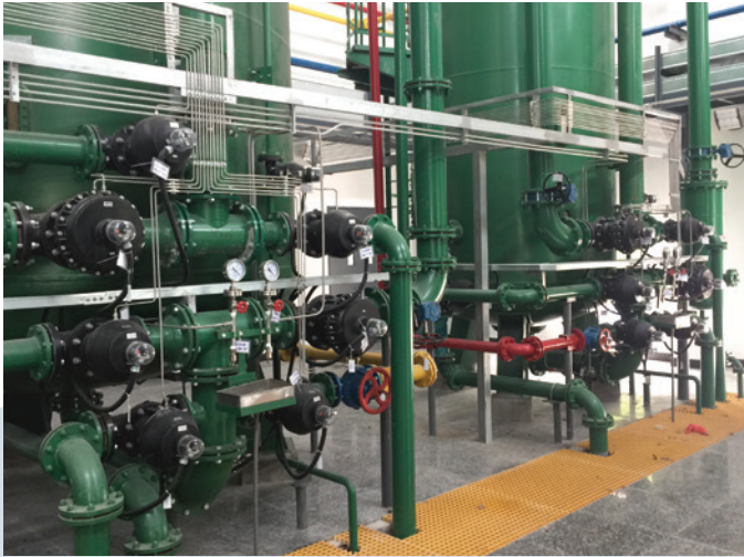
Boiled water system in coal power station
