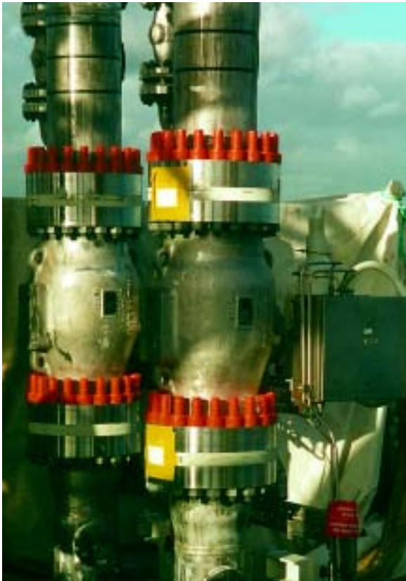
inline production chokes 10" ANSI 1500, FPSO Norway
