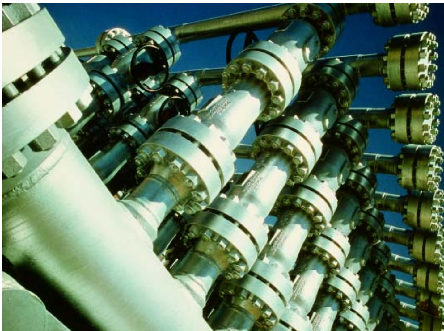
shut-off valves and non-slam check valves 6" ANSI 900 lbs, water injection manifold of a crude oil production field, North Africa
