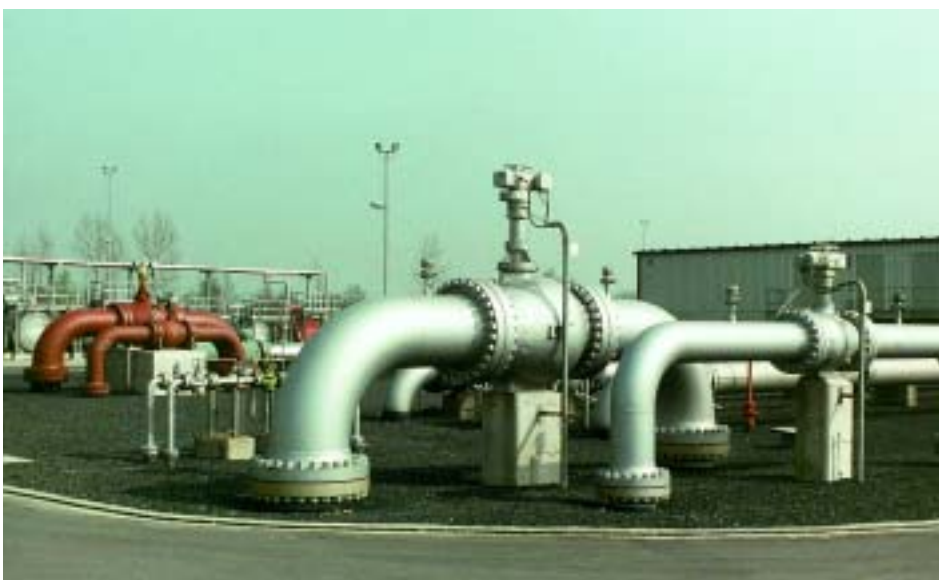
flow control valves, underground gasstorage field Germany
