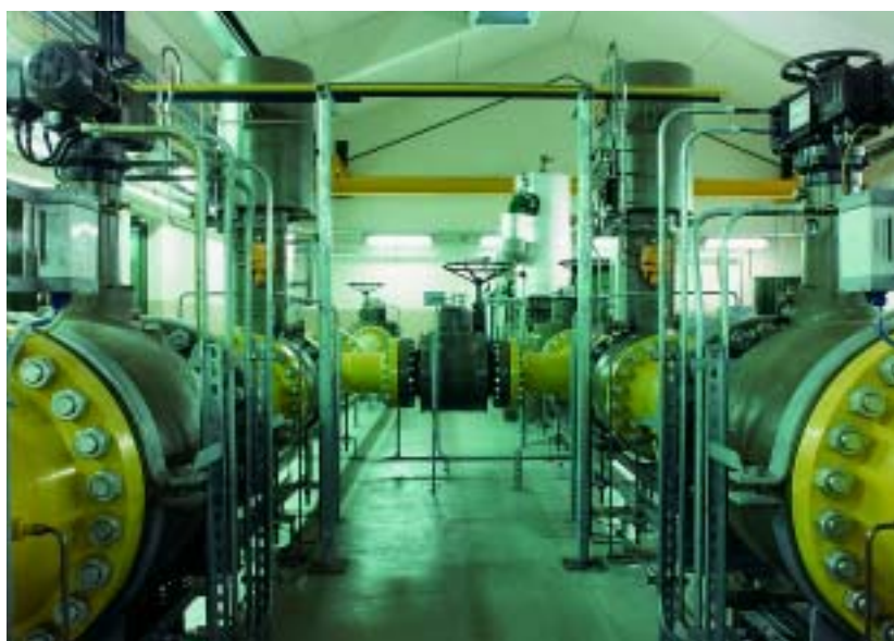
flow pressure control valves and safety shut-off valves, M & R station Germany
