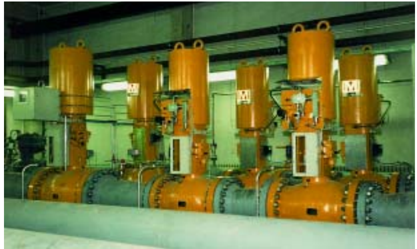
pressure control valves 20" ANSI 600 lbs and safety slam shut valves 16" ANSI 600 lbs, M & R station Germany
