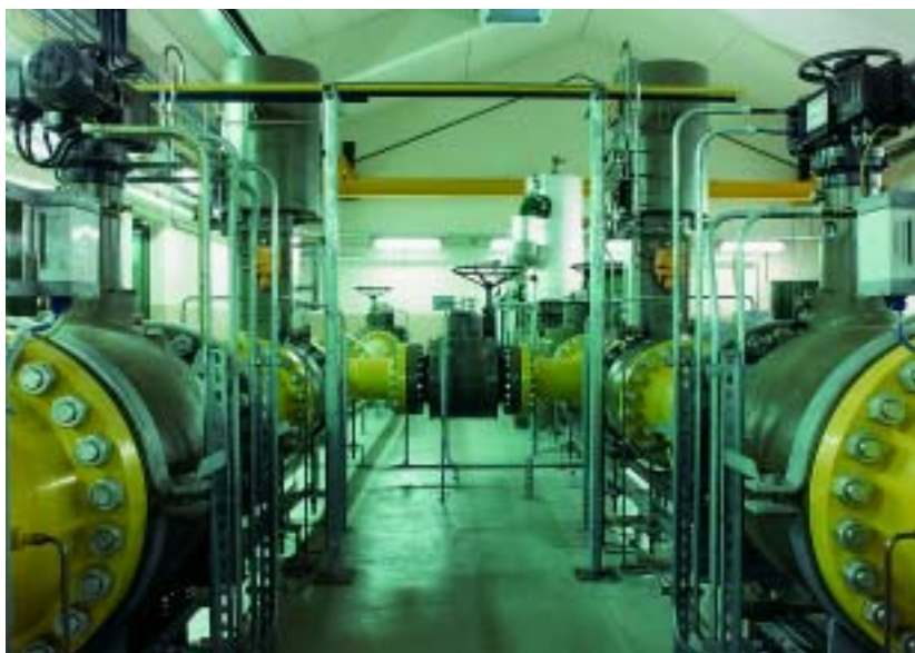
flow pressure control valves and safety shut-off valves, M & R station Germany
