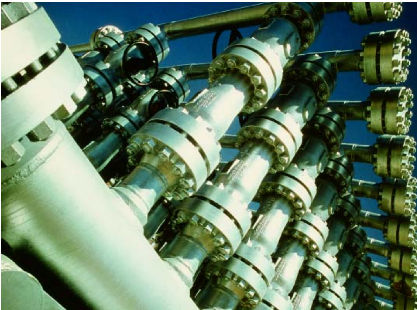
shut-off valves and non-slam check valves 6" ANSI 900 lbs, water injection manifold of a crude oil production field, North Africa
