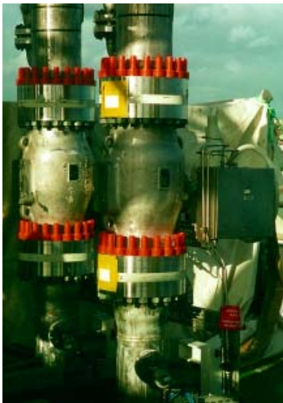
inline production chokes 10" ANSI 1500, FPSO Norway
