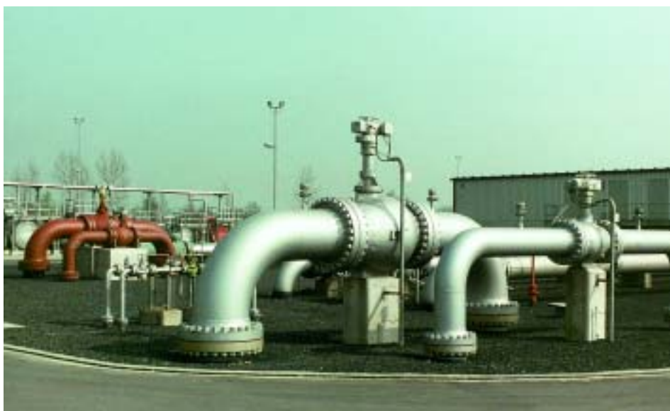
flow control valves, underground gasstorage field Germany
