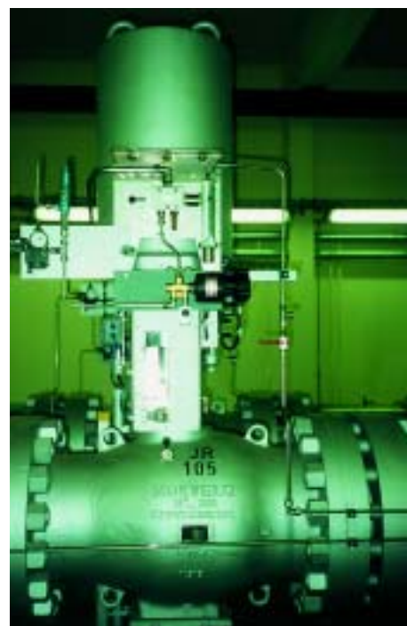
safety shut-off valve 16" ANSI 600, underground storage field Germany
