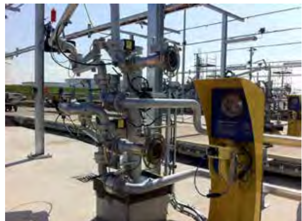
LPG loading facility
