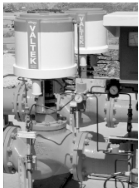
(Right) A liquid nitrogen loading facility in Australia uses two Mark One valves for its emergency fire water system.
