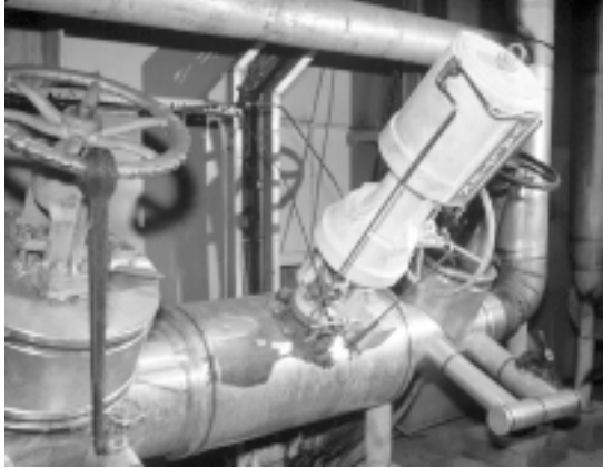
A 4-inch Mark One with side-mounted handwheel operates in a boiler feedwater system at a pulp plant.
