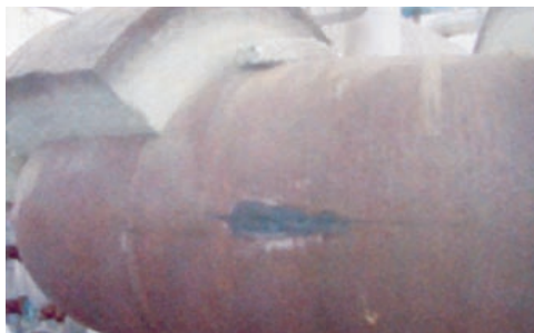
Figure 2: Illustrations of damage due to thermal cycling, often caused by poor attemperator performance.
